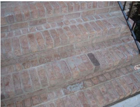
26. [A piece of masonry siding is missing above the rear wood deck.]
