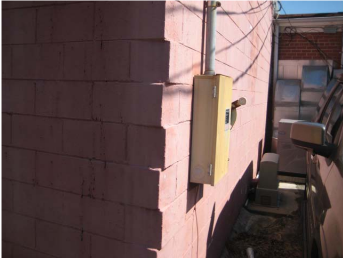
19. The two sub-panels for the branch circuits are located inside the building. The circuits for the lights and plugs are wired with copper wiring.
